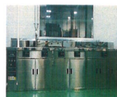
清洗线 Cleaning Line
